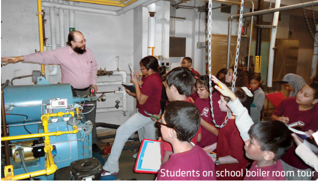
Students on school boiler room tour
